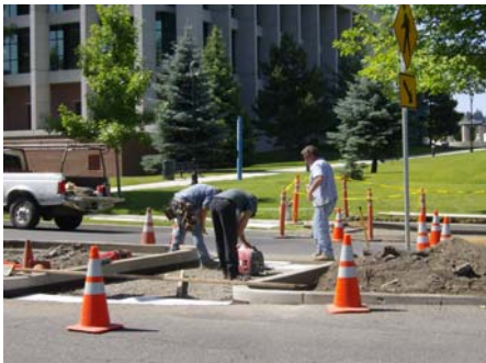
A median refuge will allow pedestrians to cross one segment of the street at a time.
